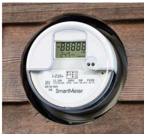
A smart meter allows you to monitor your energy usage almost in real time.
